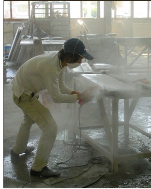
A worker at Supplier C is busy cutting edges (dry), generating a lot of dust. The face mask used is inadequate to stop quartz dust.
